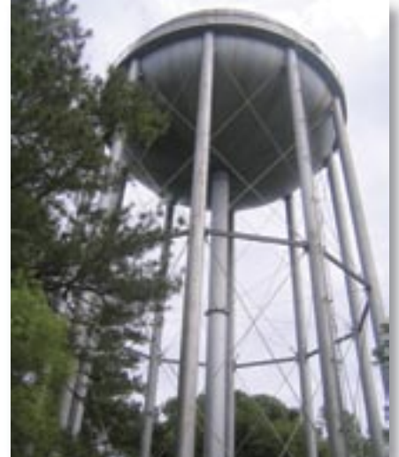
A new water tank will replace this abandoned tank on James Island.
