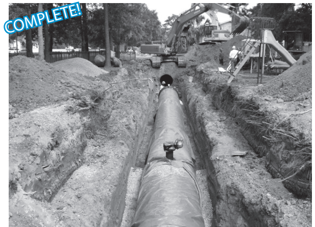
This 4-foot diameter transmission main off Murray Drive in Hanahan was also completed in 2010 as part of the 2006 Capital Improvement Program.
