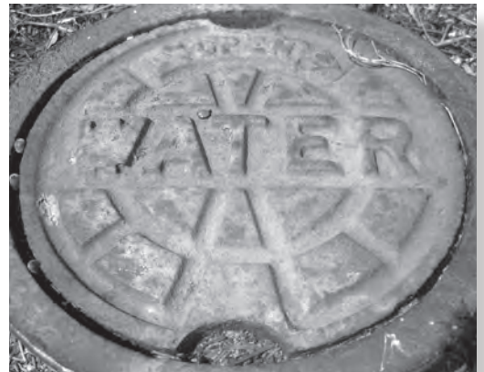
Valve cover. Water mains have valves spaced strategically along the pipeline. In the event of a leak or need for repair, crews can close valves to slow or stop the flow of water in a small stretch of pipe to limit the impact of the water outage.
